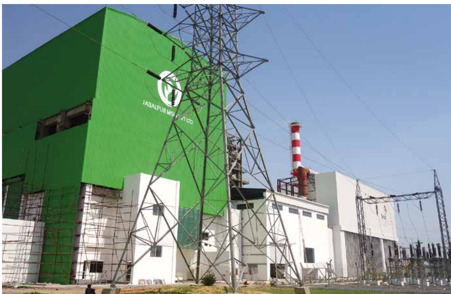
The EfW plant in Jabalpur is in operation since 2016.
