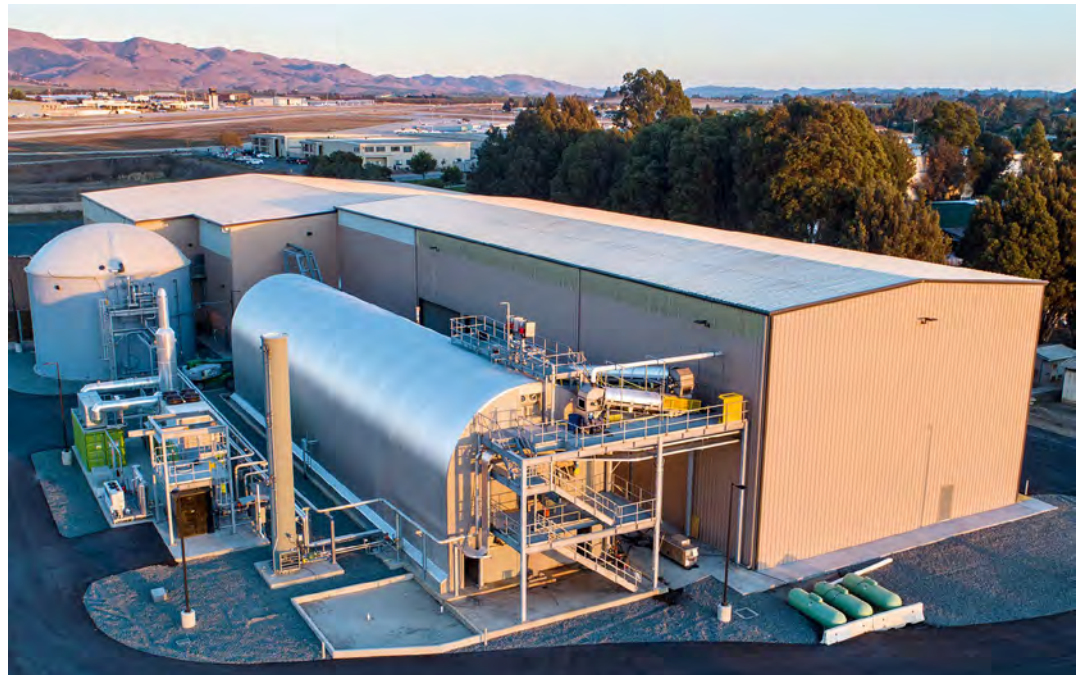
The Kompogas dry AD plant in San Luis Obispo is one of the most advanced installations of its kind in the US
